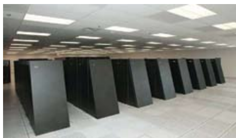
Figure 4.15 BlueGene/L Supercomputer at LLNL (The unusual slant to BlueGene/L's cabinets is a necessary design element to keep cooled air flowing properly around each cabinet's 2,000-plus processors.)
