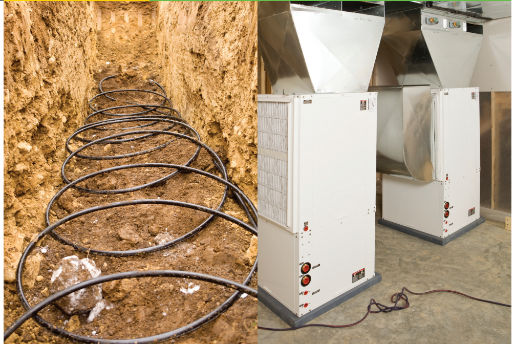
Geothermal heat pump systems, consisting of the heat exchanger (left) and the heat pump (right), heat and cool a home by transferring heat to and from the earth.
