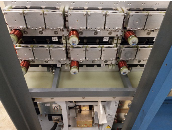
Fig. 7. Installed solid state switch modules. The system was designed for 50 kA; it was populated and tested with modules for 25 kA.
