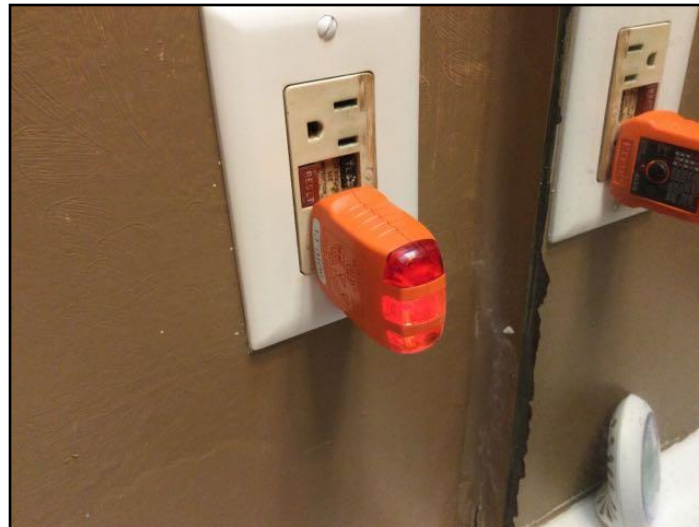
34. Test faulty on GFCI/GFI (Ground Fault...
