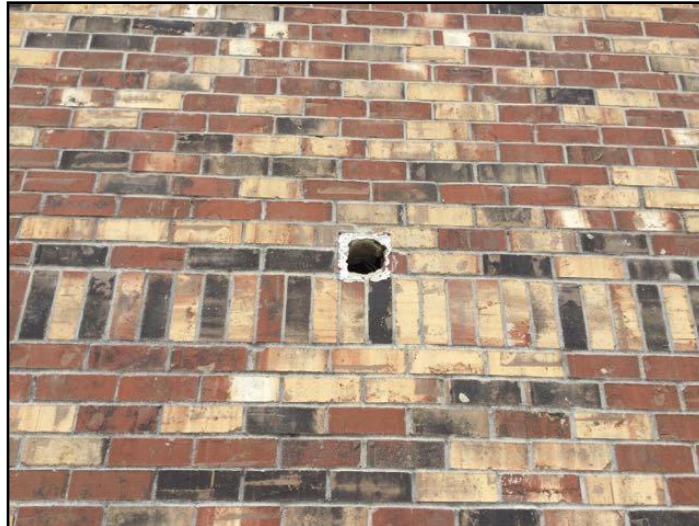
50. Missing exterior cover
