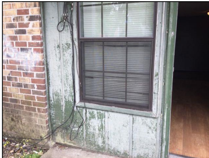
1. Paint or stain - needed
