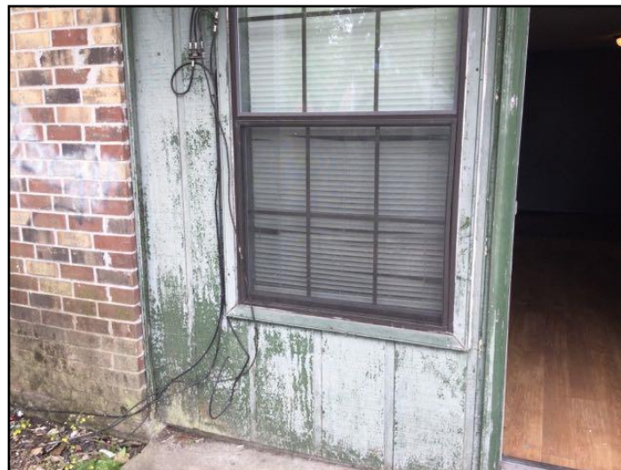
23. Paint or stain - needed
