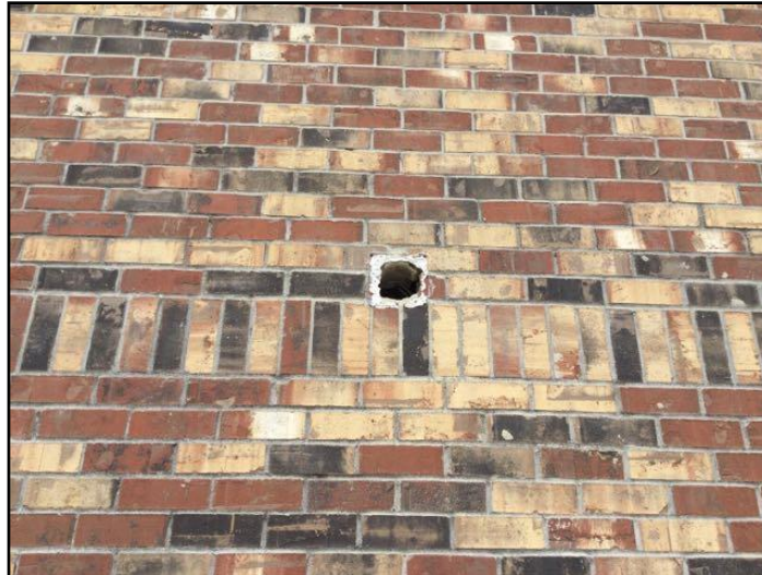
22. Missing exterior cover
