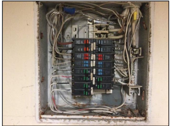
29. Breakers - laundry room
