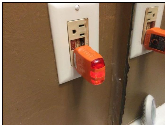
7. Test faulty on GFCI/GFI (Ground Fault...
