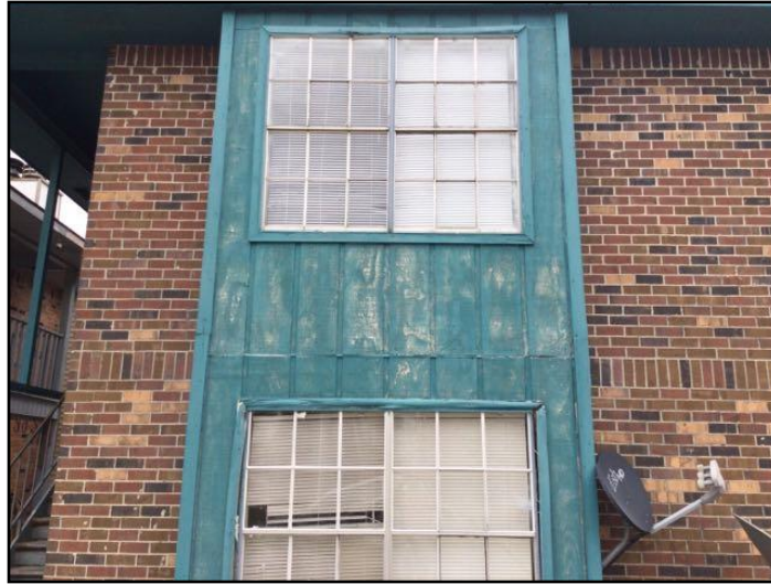
26. Paint or stain - needed
