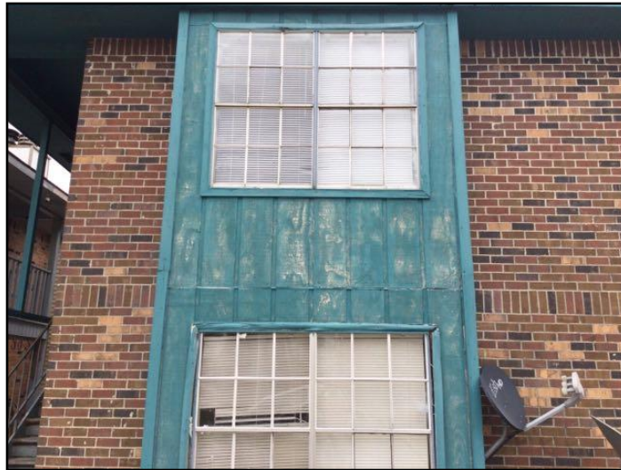
2. Paint or stain - needed
