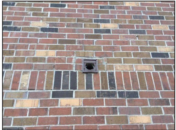
24. Missing exterior cover
