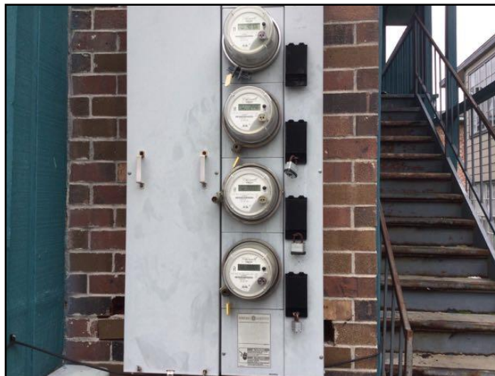
30. Breakers - exterior wall
