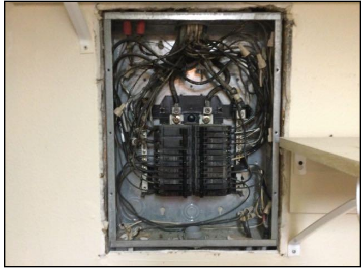
32. Breakers - laundry room
