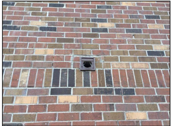
54. Missing exterior cover
