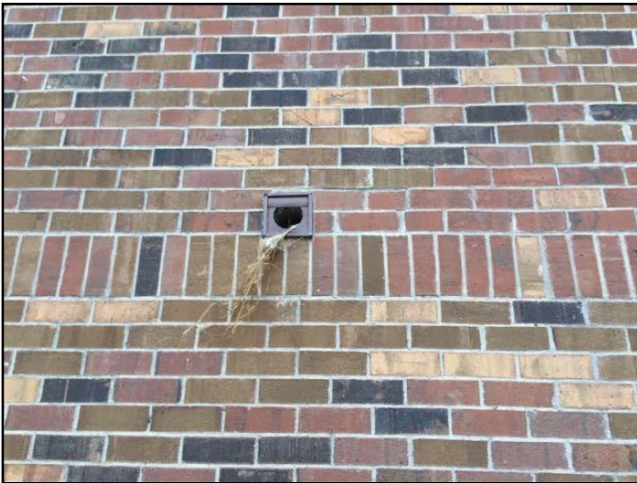
53. Missing exterior cover
