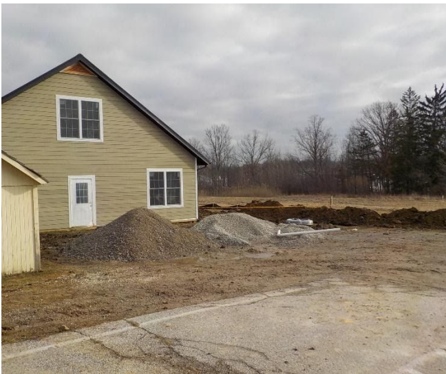
Trenches on the east and piles of dirt are becoming familiar sights at the farm
