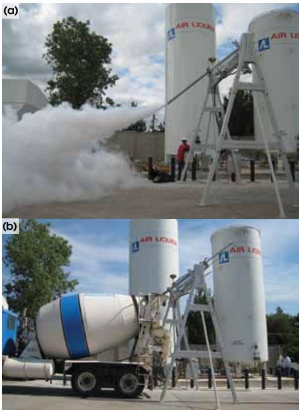
Fig. 2: The CryoCrete™ automated LN cooling system developed by Air Liquide Industrial U.S. LP: (a) during injection testing and (b) just before cooling of a load of concrete in a truck
