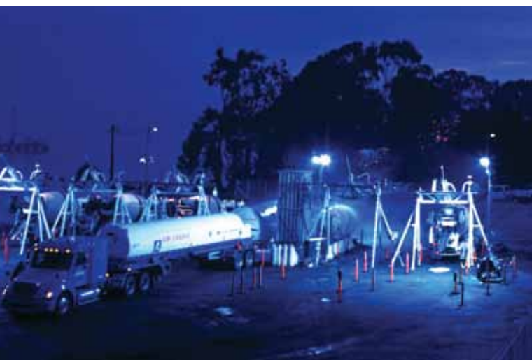
Fig. 1: Night construction of the new Oakland Bay Bridge, San Francisco, CA, using an LN cooling system
