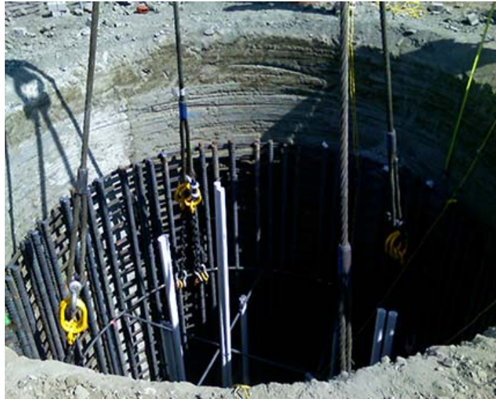
Fig. 1. Cooling pipes (white PVC) in a 12-ft diameter drilled shaft prior to placement of the concrete.
