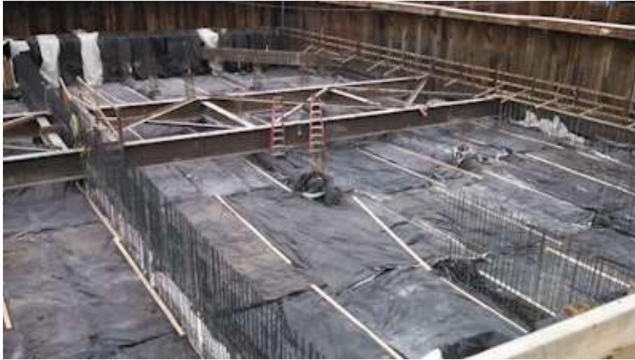
The contractor did a careful job of insulating the concrete to prevent temperature differentials greater than 35°F. However the vertical rebar must also be insulated because steel is a good conductor of heat. Photo Credit: John Gajda
