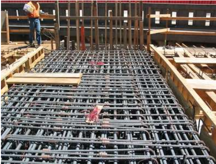
Shown here are temperature sensor wires. The thermal sensors are wired to locations all over the rebar reinforcement.
