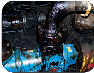
Fuel Oil Pumps
