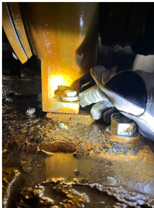
Photo 4 - Pump Valve Mounting Hardware Discovered Loose
