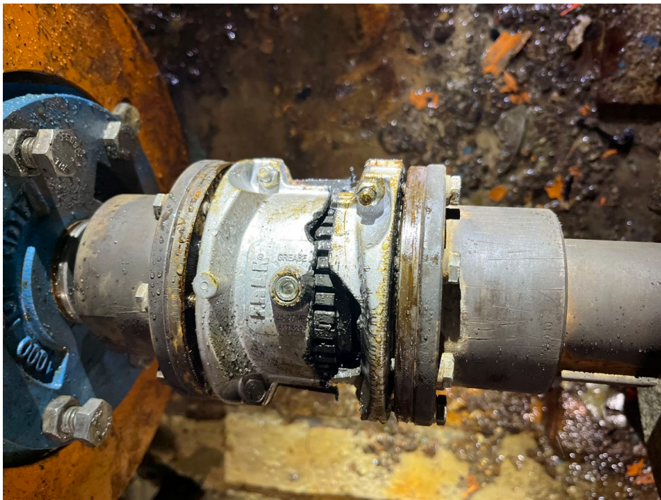
Photo 2 - Pump Coupling Bending Fracture
