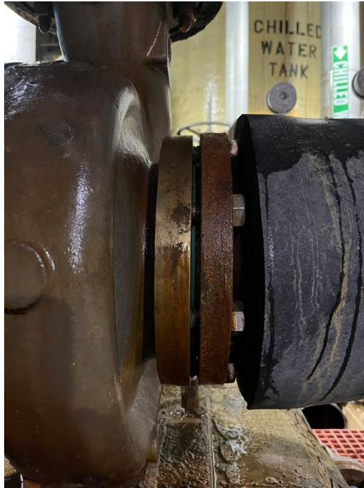
Photo - 5 Suction Flange Visibly Misaligned
