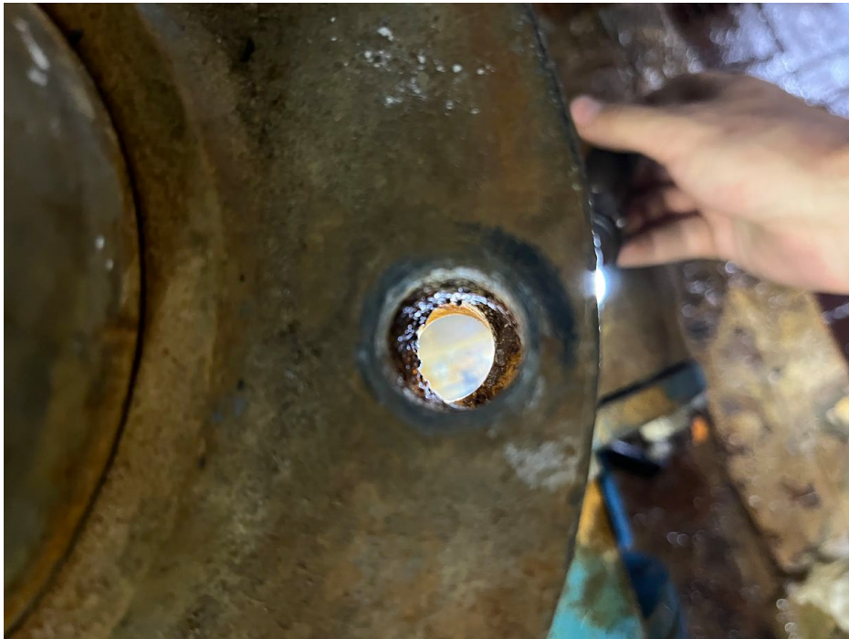
Photo 7 - Pump Discharge Flange Misalignment
