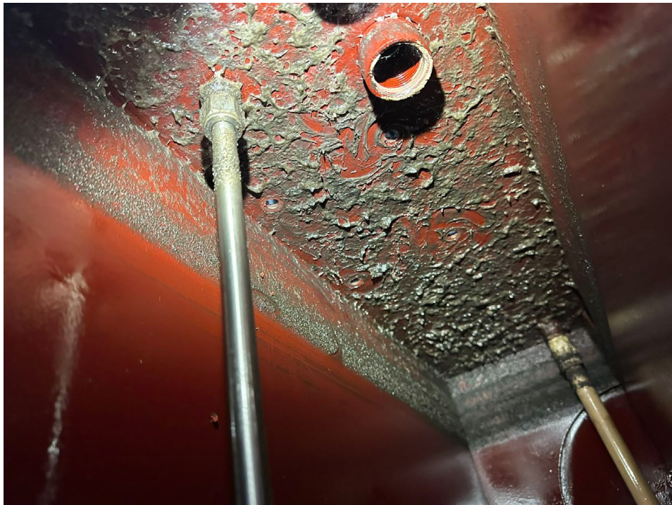
Photo 18 - Chipper Lube Tank Top - As Found Condition
