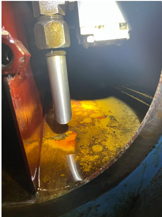
Photo 17 - Chipper Lube Tank Bottom - As Found Condition
