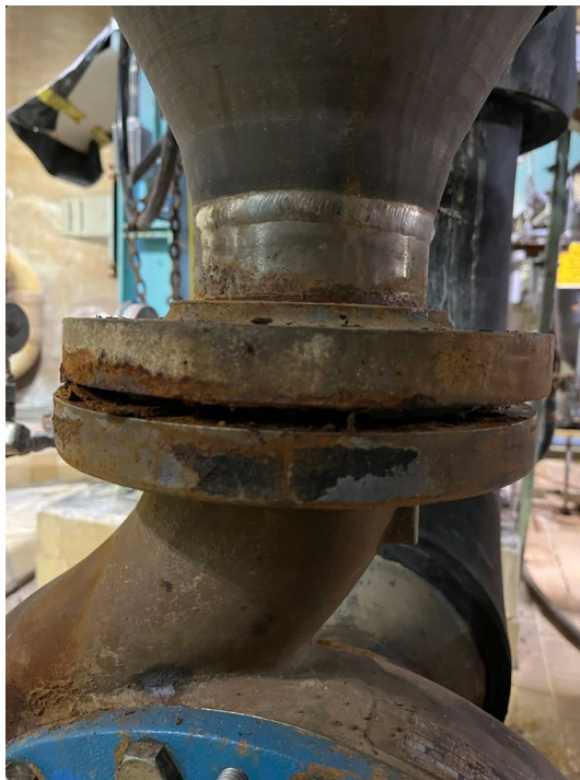
Photo 6 - Pump Discharge Flange Misalignment
