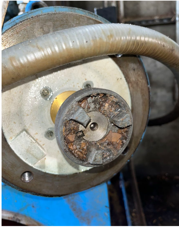
Photo 21 - Chipper Lube System Pump Coupling Damage
