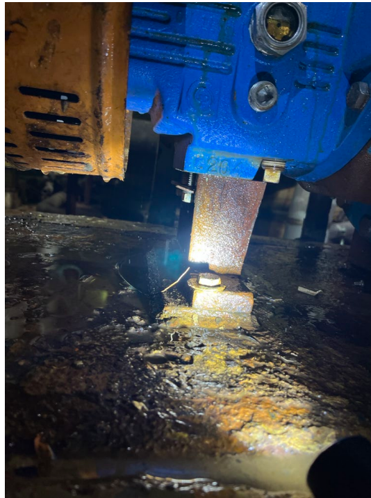
Photo 3 - Pump Pedestal Mounting Hardware Discovered Loose
