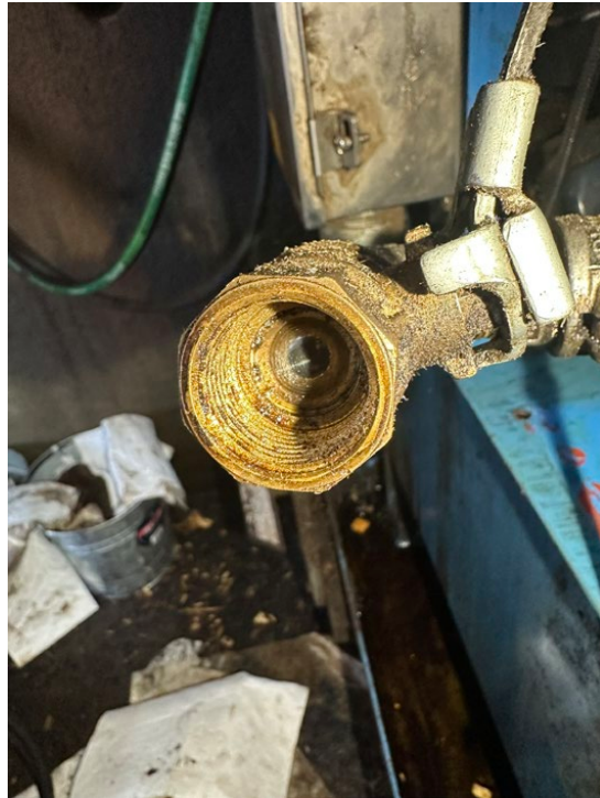
Photo 19 - Chipper Lube Tank Inlet Connection - Contamination
