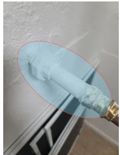
It looks as though the main water pipe to the house is older galvanized steel.
