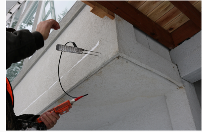
This photo shows an example of moisture probes looking for moisture in a synthetic stucco system.
