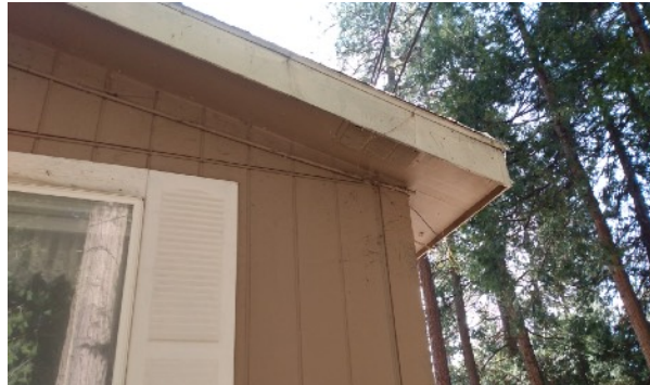
Closed in eaves, no gaps
