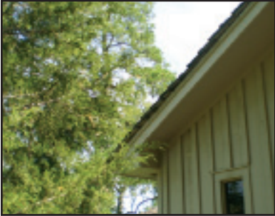
Overhanging branches can drop embers onto a roof.
