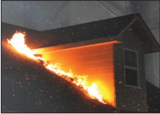
Debris can build up in corners, providing fuel for embers. Photo by Institute for Business and Home Safety Research Center.
