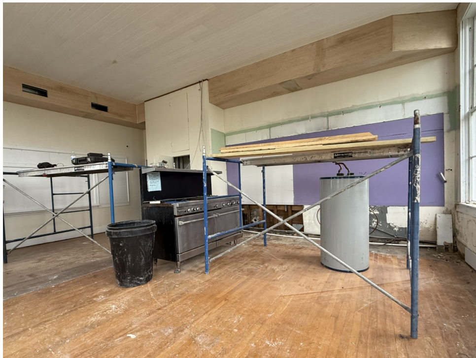
The vintage commercial stove stands in the center of the historic school-house's kitchen. Framed by scaffolding and stripped walls, the quiet space pauses in mid-transformation as modern renovations breathe new life into the space. (Photo provided by Jim Sylvester.)
