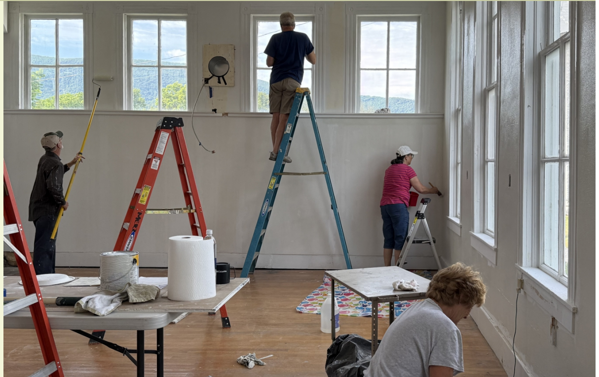
A fresh coat of paint is applied to the walls of the kitchen by Jim Sylvester, Steve Merz, Lisa Merz, and Roxanne Campbell (l. to r.). (Photo provided by Jim Sylvester)
