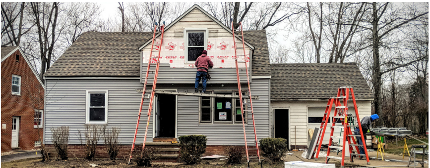
Single-Family Infill Home built by The Cuyahoga Land Bank Image Source: Cuyahoga Land Bank, South Euclid, Ohio
