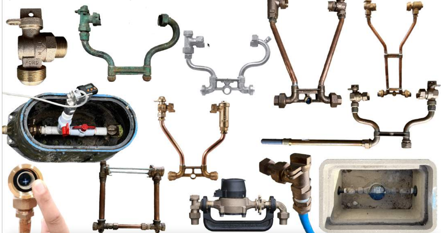
Figure 34. Various Curb Box Meter Settings.
