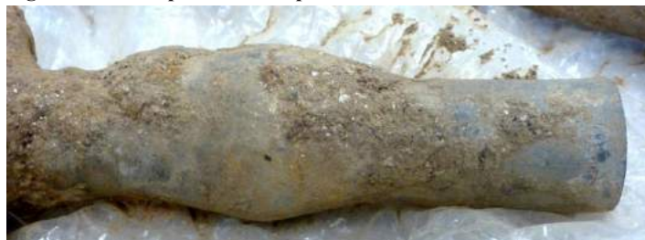
Figure 1. Lead Pipe at Curbstop.
