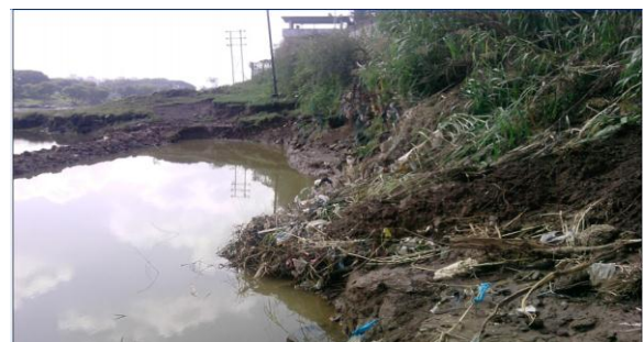
FIG 8- Bank erosion at Ordinance factory, Kirki, Pune
