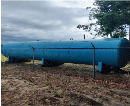
Exterior of the Hydropneumatic Tank (HPT)
