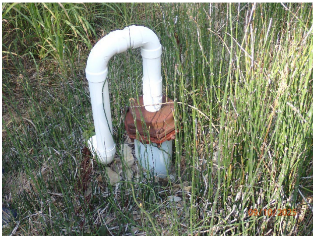
Valve pump at toe
