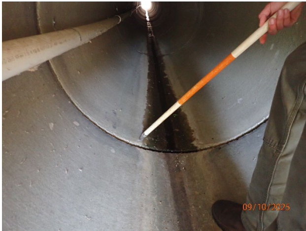
Principal spillway outlet (note water flowing through joint)
