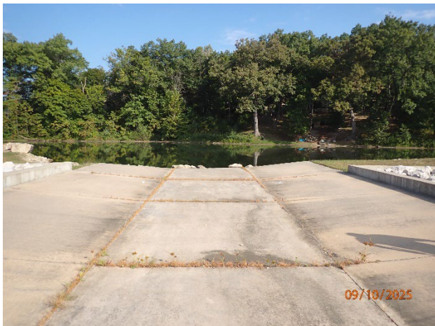
Auxiliary spillway – looking upstream (note vegetation in joints)
