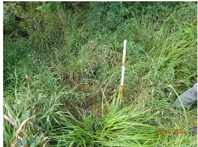
Right groin (note seepage)
