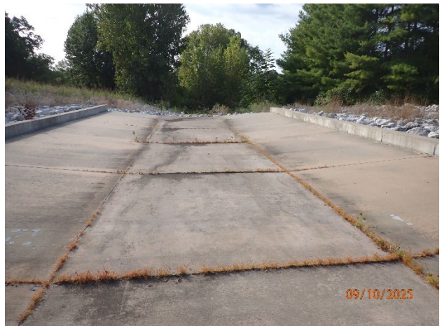
Auxiliary spillway – looking downstream (note vegetation in joints)
