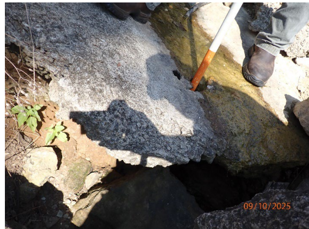
Principal spillway outlet – note undercutting of concrete
