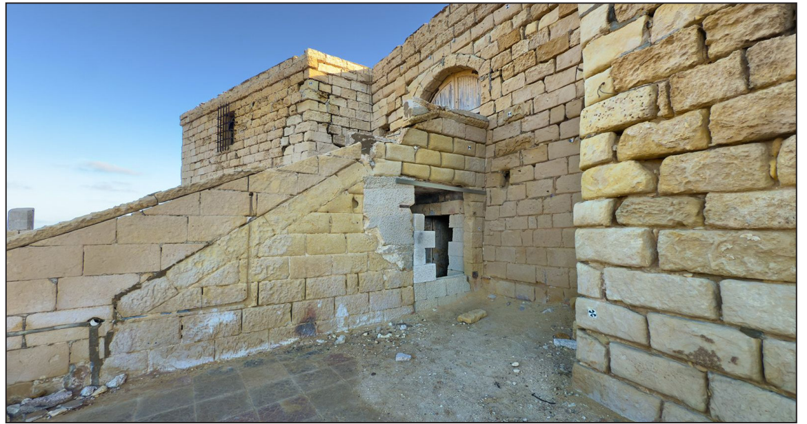
In the 1970s, the Battery was handed over for private use as a nightclub and disco. Significant damage was inflicted through excavations and later accretions, which severely compromised the fabric of the building
