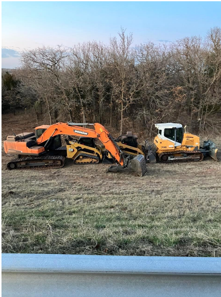
Basin Scrubbed Below the Dam
