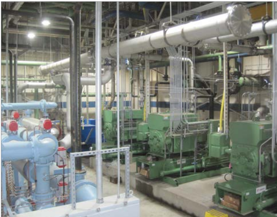
The upgraded compressed air system at KTP has reduced energy consumption by approximately 9.2 GWh. (Photo courtesy of Universal Compressed Air.)
