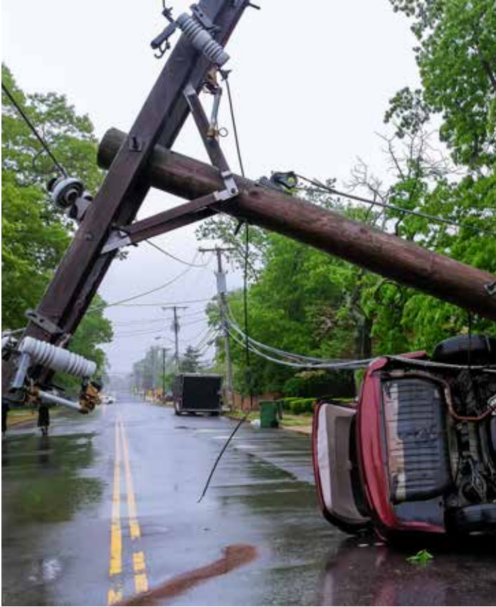
Ill. 5 (above left): Severe weather can bring down power lines.
