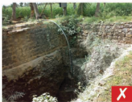
Open wells without fencing
