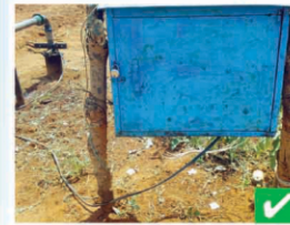
Well maintained electrical panel board
