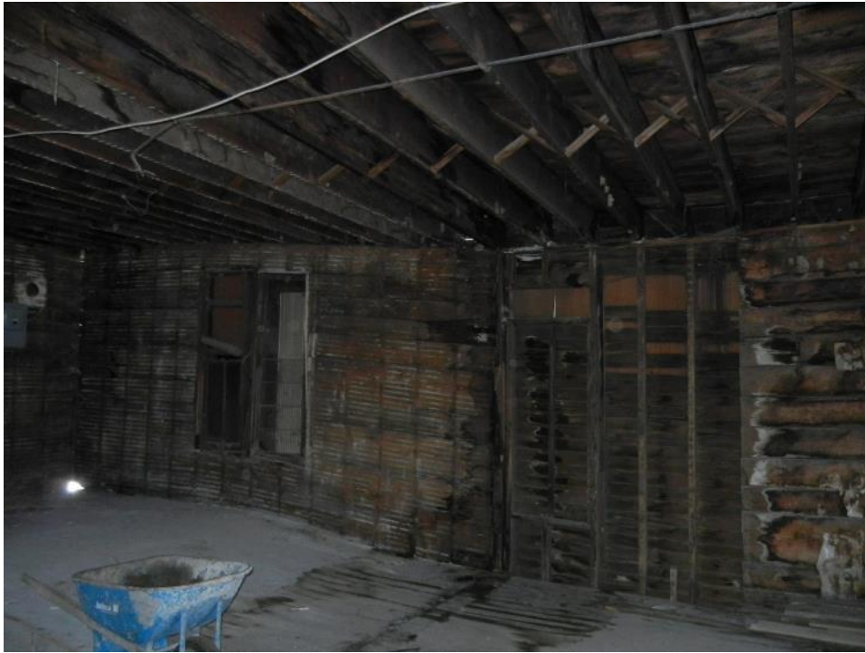
Photo 52: Second floor, south section, wall and ceiling
