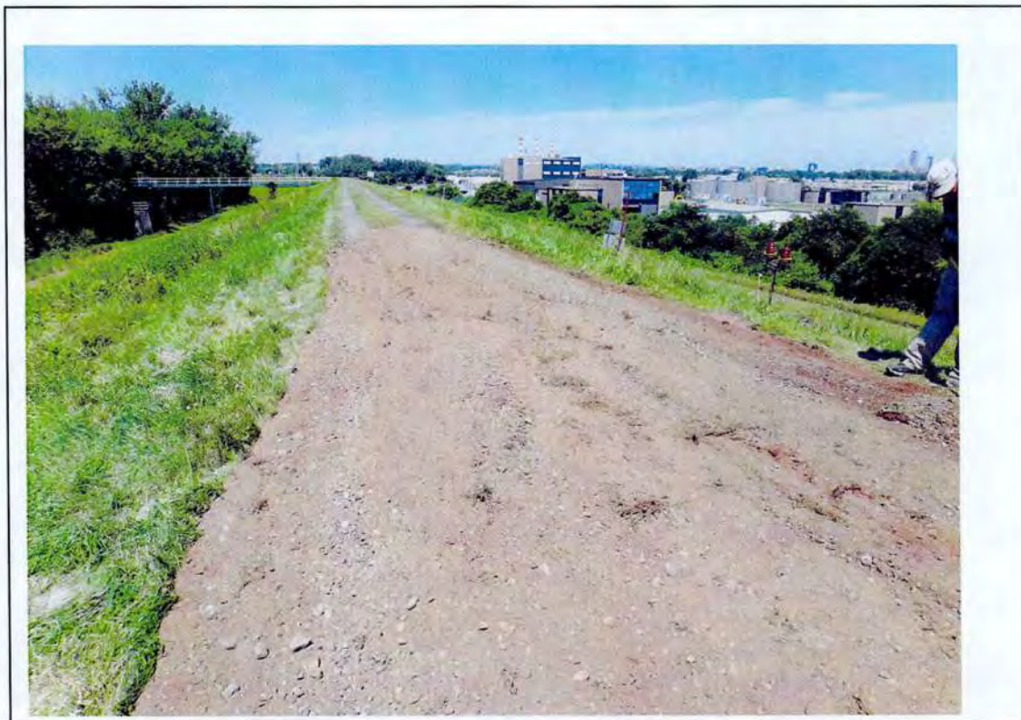
Picture # 2 of 2 Taken By: ERC I 929 Date: 6/30/2012 Description: This is a photo of the flood control dyke after clean-up.
