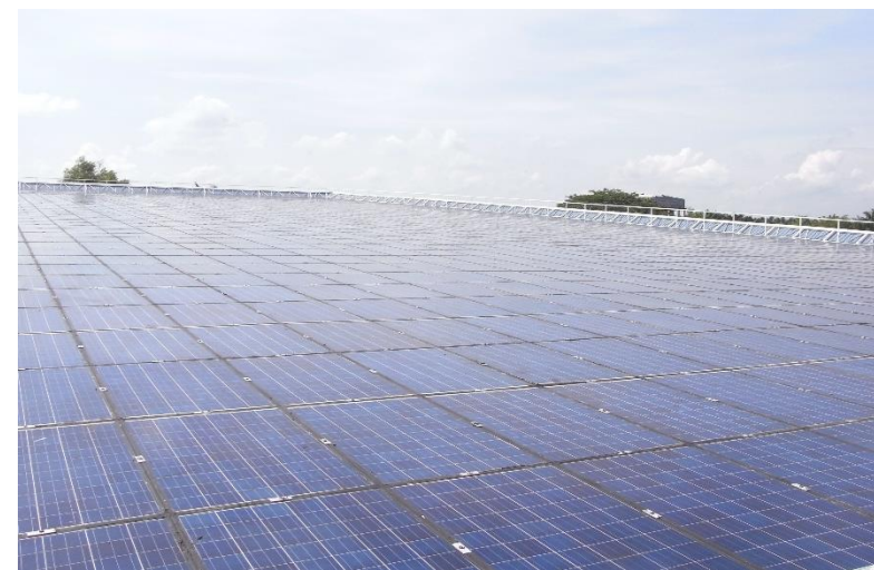
425kWp FiT @ Kuala Kertih 2012
