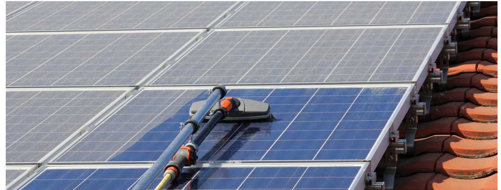
Solar Modules Cleaning
