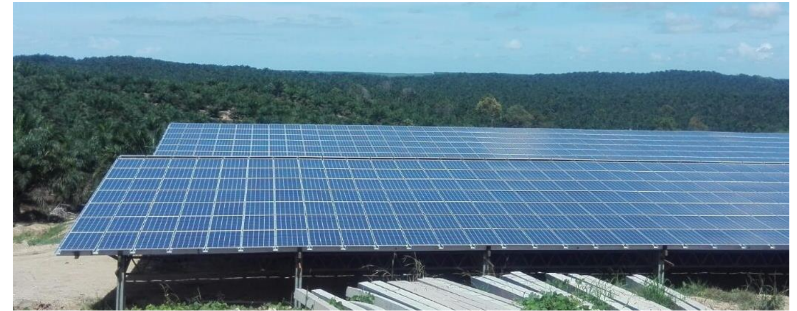
1MWp FiT @ Sandakan 2016
