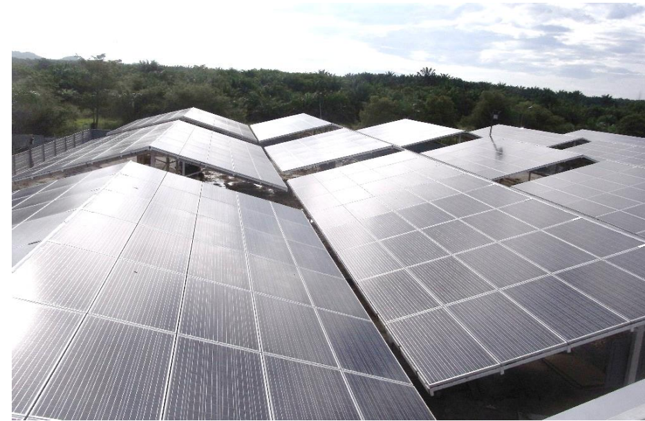
425kWp FiT @ Kuala Kertih 2012
