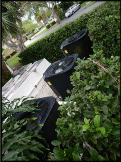
pool/spa equipment & heater
