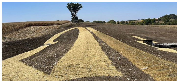
Earthen dam constructed on a tributary to the Redwood River (BWSR Snapshot)
