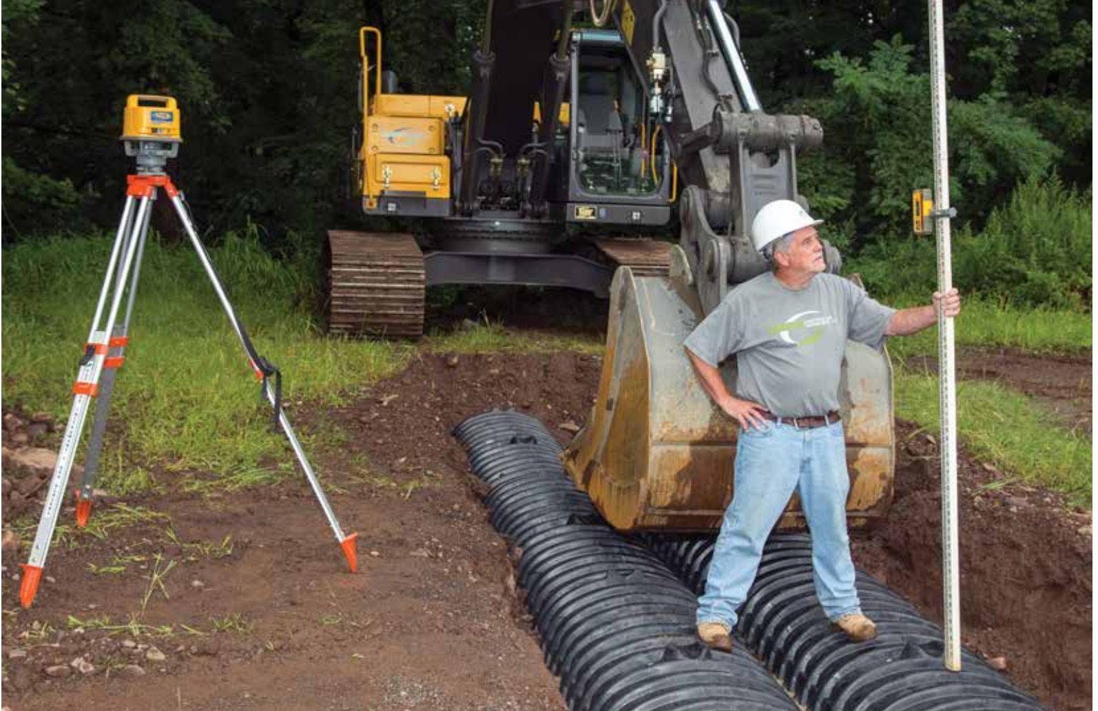
ABOVE: Wayne Green uses a Spectrum LL500 laser/target (Spectra Precision) to confirm the proper height of a double row CULTEC Contactor 100 chambers at a work site.
