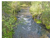
Photos to the Left: These rock and log v-weirs were built in 1997 and these photos were taken in the summer of 2008. You can see that the moss and shoreline cover has made it difficult to tell whether they were man-made or they are natural. This is what we had all hoped for!
