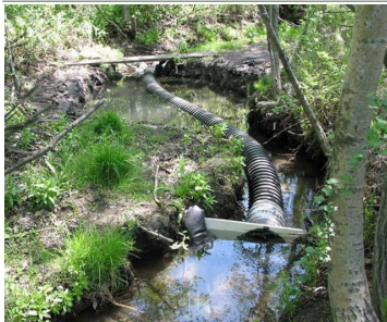
Above: A flow by-pass pipe is placed into the stream channel to isolate the work area and allow clean water to be diverted around the pool excavation site.
