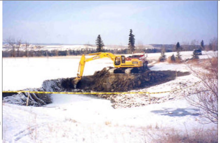
In 1999, heavy equipment was brought in to excavate the lower Mitford Pond. An area on the north end of the lower pond was deepened to a depth of 13 feet.
