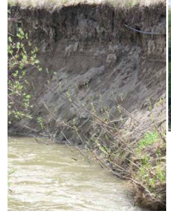
Left photo: This photo shows an eroding stream bank on BH Creek, just after planting. This was a major soil and clay loading site, on the creek channel.
