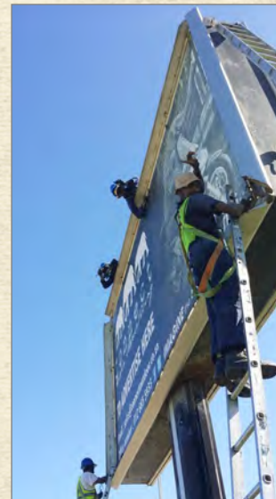
Mom and I passed by some men putting up a billboard. Just ladders on unstable ground to get to the top. No safety straps. Probably 30 feet or more high.
