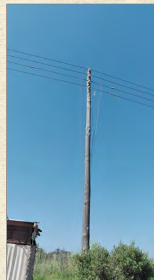
People that live in the shacks need electricity. They will run wiring down from the power lines that goes to the government houses and "steal" electricity. The wires just run on the ground and over to the shacks.
