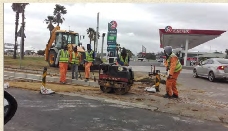
Work continues on an intersection that was begun over 6 months ago. Most work is pick and shovel. In the USA, I'm guessing it would be a two week job.
