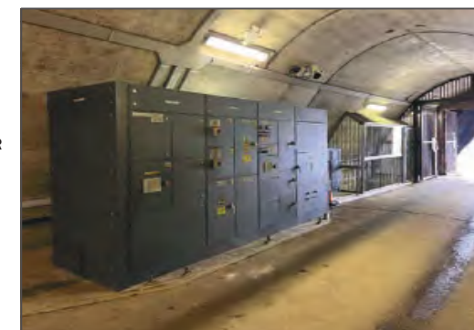
FINISHED ELECTRICAL BOX ON LOCATION
