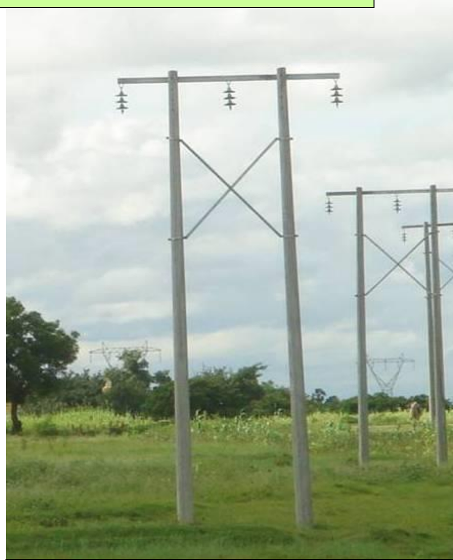
Single H-Pole Structure Suspension
