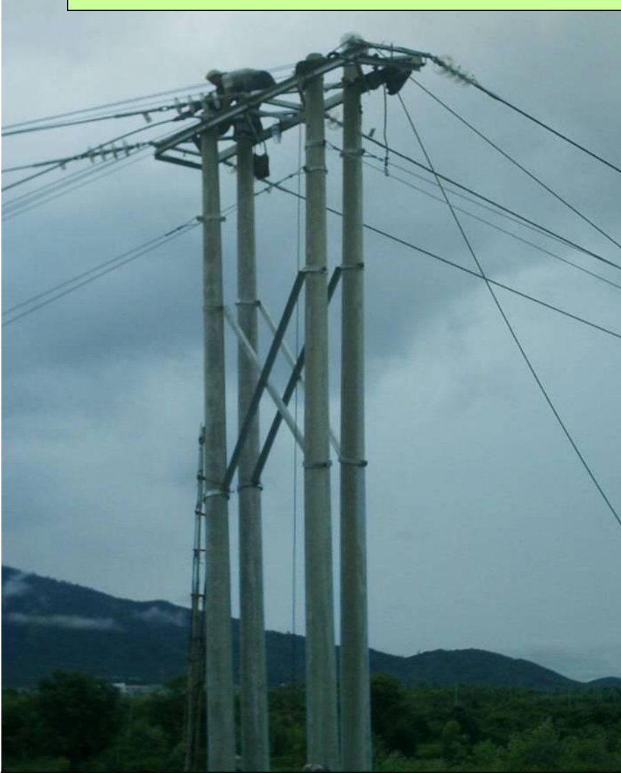
Double H-Pole Structure Tension
