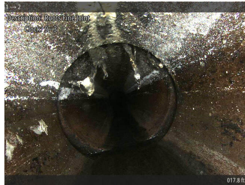
Roots Fine Joint at 017.8 ft, 9 - 3 o'clock
