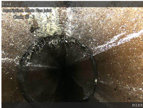
Roots Fine Joint at 012.8 ft, 10 - 2 o'clock
