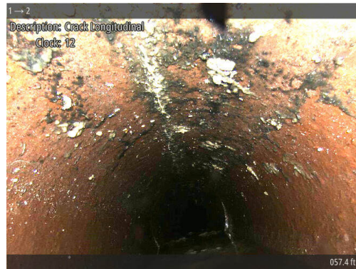
Crack Longitudinal at 057.4 ft, 12 o'clock
