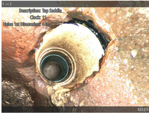
Tap Saddle at 023.0 ft, 11 o'clock
