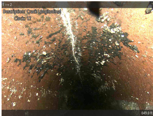
Crack Longitudinal at 049.0 ft, 12 o'clock
