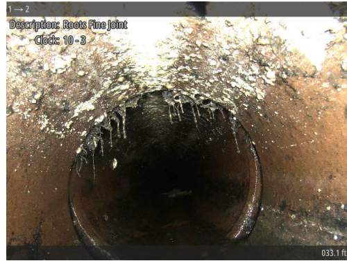
Roots Fine Joint at 033.1 ft, 10 - 3 o'clock
