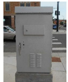
Small door is PD access
