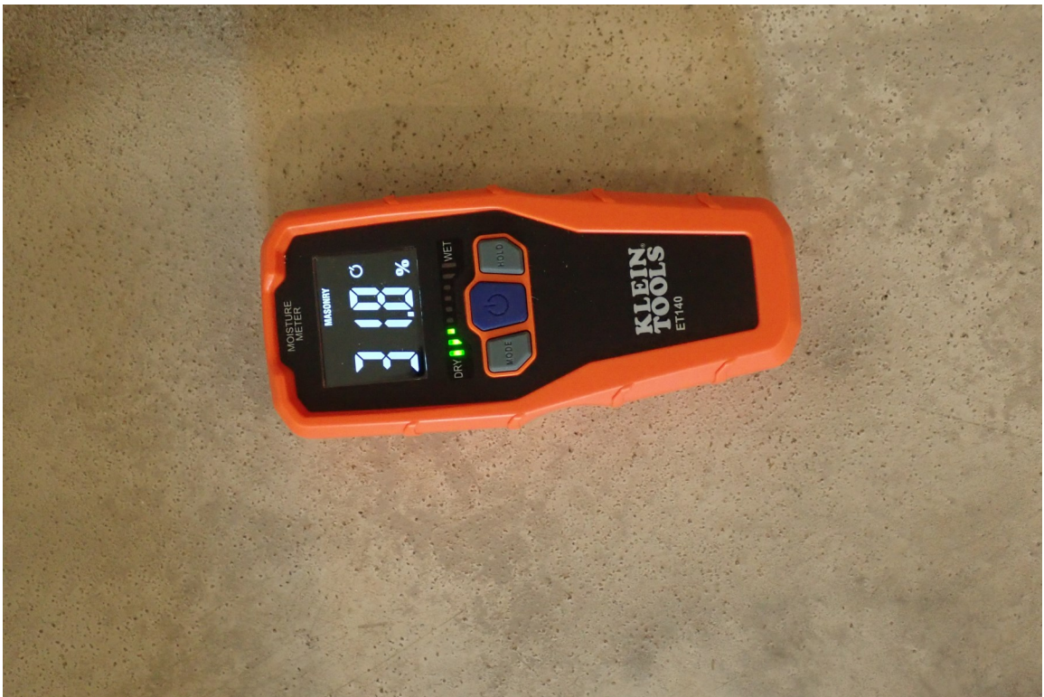
Figure 2 Concrete moisture reading at previous repair location
