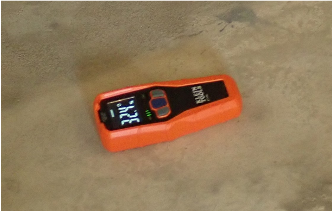
Figure 3 Concrete moisture reading at previous repair location
