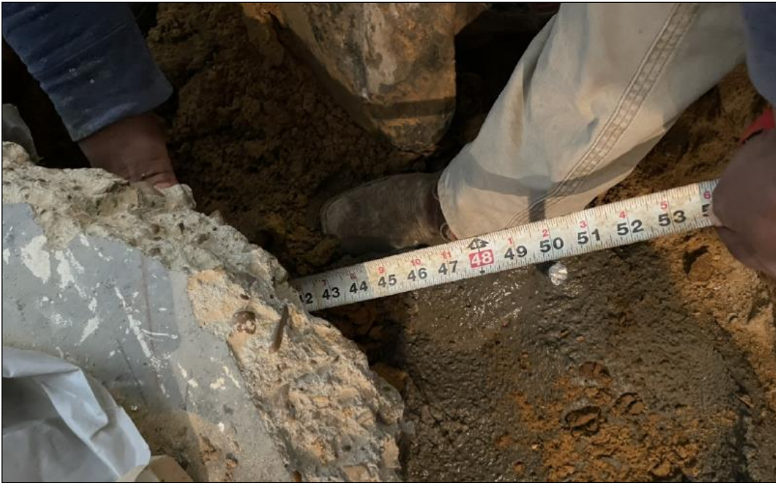
Figure 2 - Photograph taken by homeowner during plumbing repairs, which required demolition of main slab. Tape measure is inserted in area of required 30-inch by 30-inch footing.
