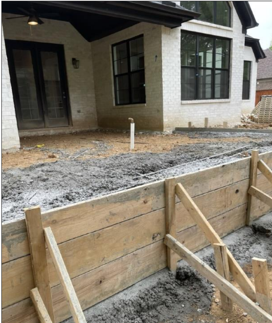
Figure 4 —Photograph taken by homeowner during placement of OLA patio slab. Steel reinforcement is observed to be lying on the ground.
