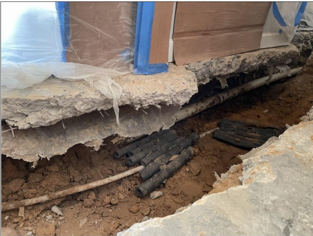
Figure 3 —Photograph taken by homeowner during plumbing repairs, which required partial demolition of main slab. The Welded Wire Reinforcement (WWR) is observed to be lying directly on top of vapor retarder.
