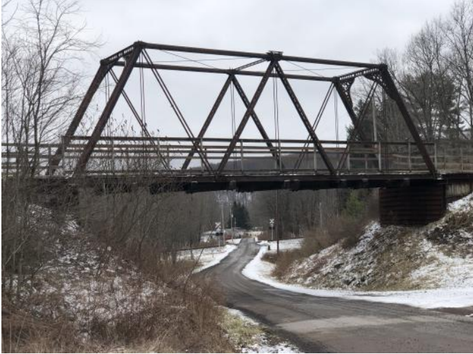
The neat little truss bridge is actually the ex-Western Maryland (now a bike path), the B&O is the line in the distance. This is heading up from Meyersdale PA to the tunnel.
