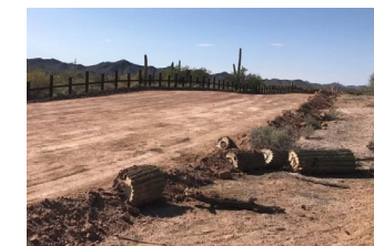
Photo of destroyed burial site at Organ Pipe National Monument for construction of border wall
