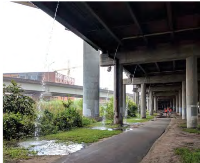
Current Site Conditions: Runoff from the overpass
