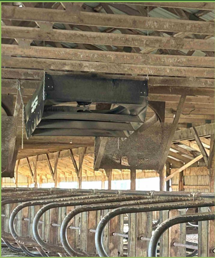
One of four Air Blaster fans installed in the free-stall barn
