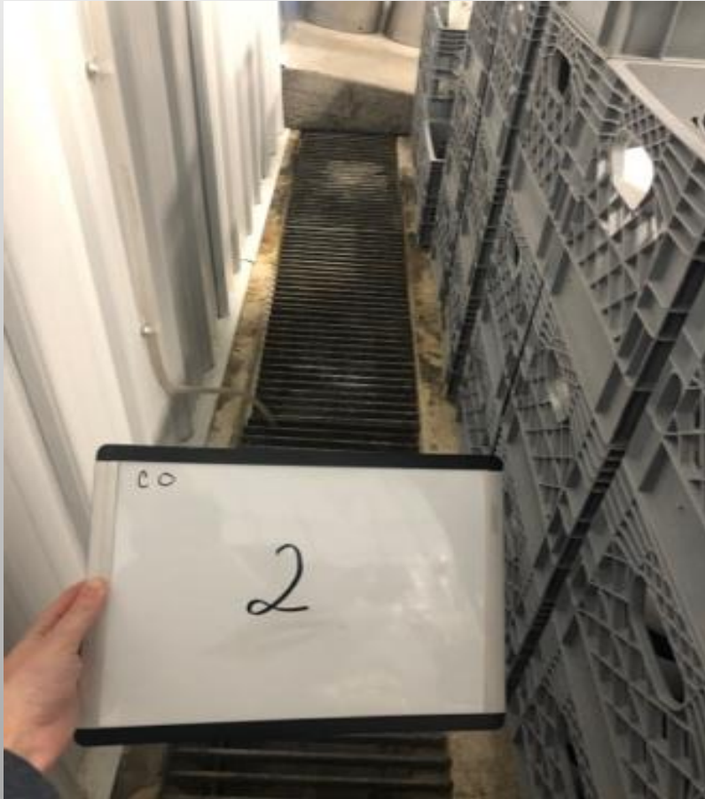
Cooler drain (CO2)
