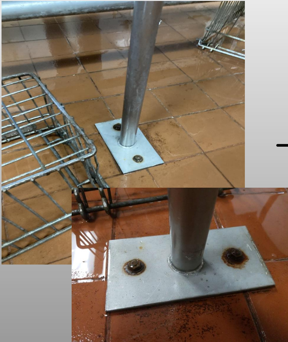
Before corrective action
