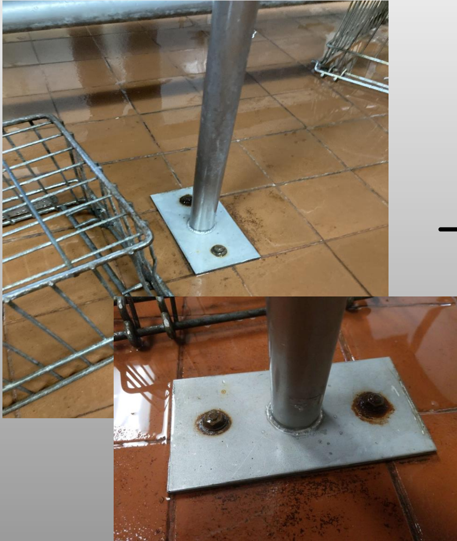
Before corrective action
