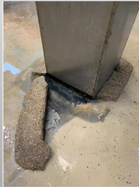
Before corrective action
